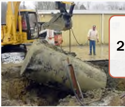
Underground Storage Tanks
